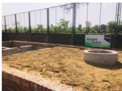
Bio Gas Plant
