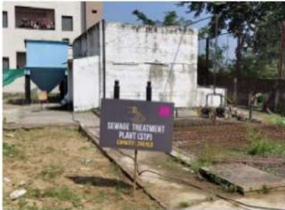
sewerage treatment plant
